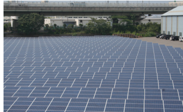
Photovoltaic power generation system at the Izumiotsu Plant
