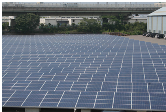
Solar panels at the Izumiotsu Plant
